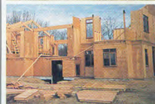
Top: Components fabricated at Deck House's Acton, Massachusetts, facility are shipped within four weeks. Middle: Typically, three shipments are scheduled; components arrive on site as needed. Bottom: Materials are arranged in order of use at the site.
